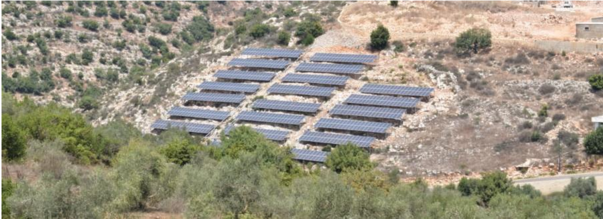
Figure 2: 250 kWp system implemented at Kabrikha, South Lebanon
